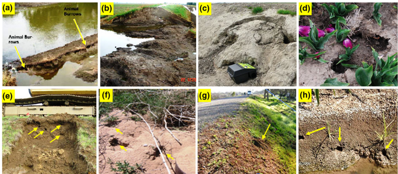
Fig. 1 Wildlife damage to earthen structure: (a, b) Pin Oak levee failure due to muskrat burrows in Winfield, Missouri [104]; (c, d) earth dikes near tulip fields damaged by rats in the Netherlands [35]; (e, f) deep cavities and surface burrows of rodents [20]; (g) animal burrows in highway embankments [20]; (h) crayfish damage in the banks of the Nile River in Egypt [133]
